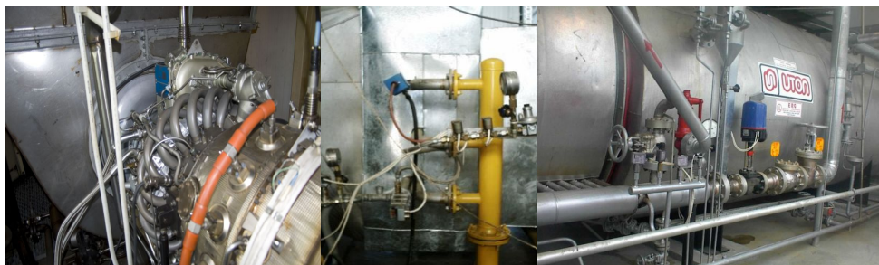
Fig. 2. ST 18 gas turbine (left), afterburning installation burner (centre) and heat recovery steam generator (right) at 2xST 18 Cogenerative Power Plant
